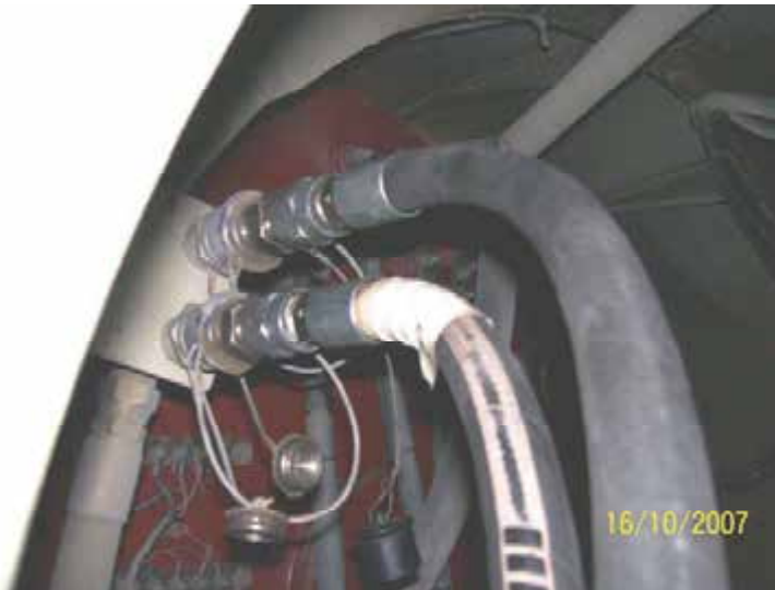
Manifold close to tub access door with suction line from bottom of wheel motor and return line back to top for ideal circulation
