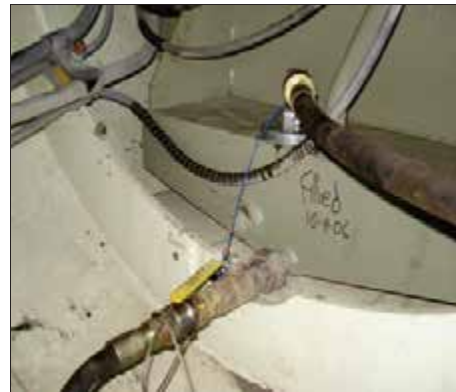
Typical filtration connection points on a Komatsu 830E wheel motor oil reservoir
